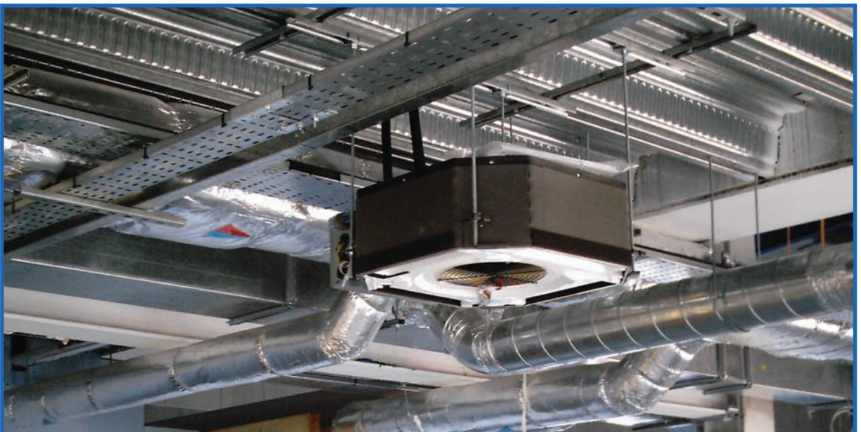
TYPICAL EQUIPMENT WITHIN CEILING VOID
